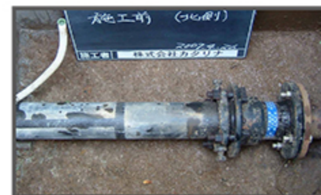
[Water supply line]
