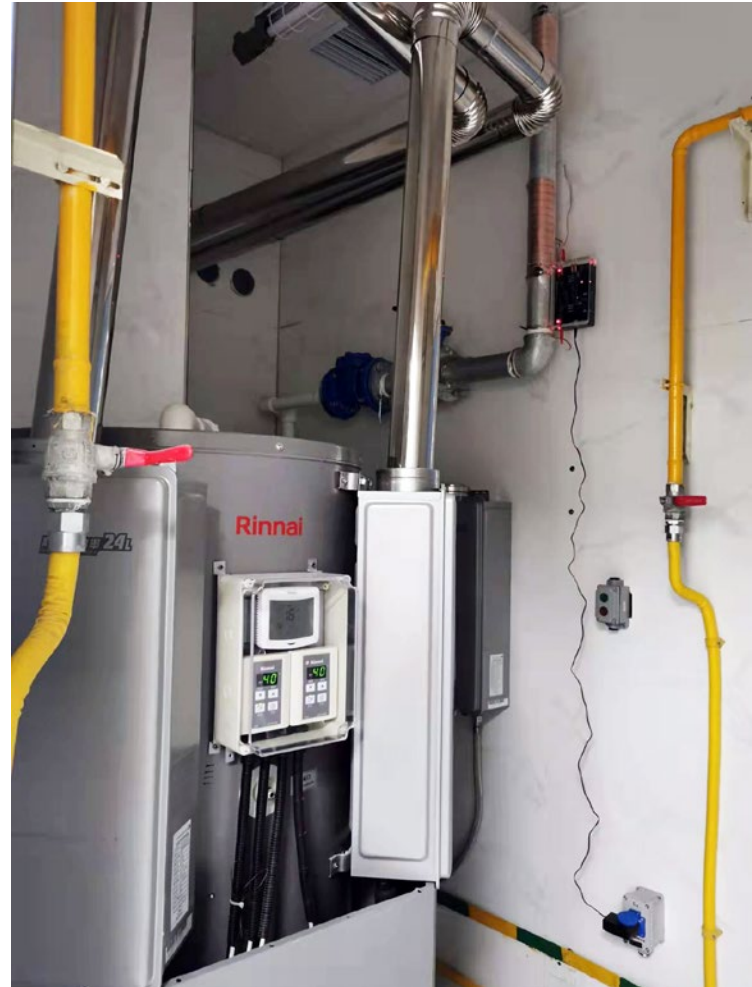
Vulcan S10 treats the canteen hot water system.
