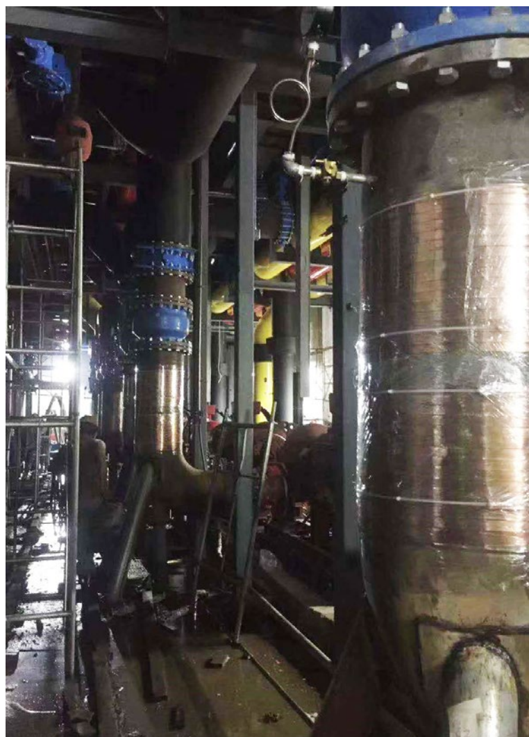
6 x Vulcan S500 were installed on the pipelines of the central air-conditioning circulating water system.
