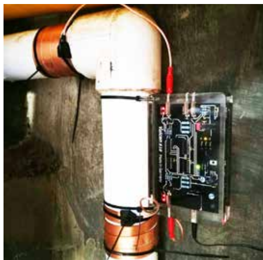
Vulcan S10 installed on the main water outlet pipe.
