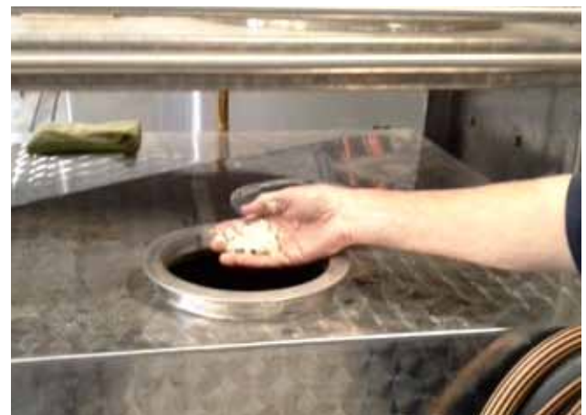
Scale deposits removed after installing the Vulcan 3000
