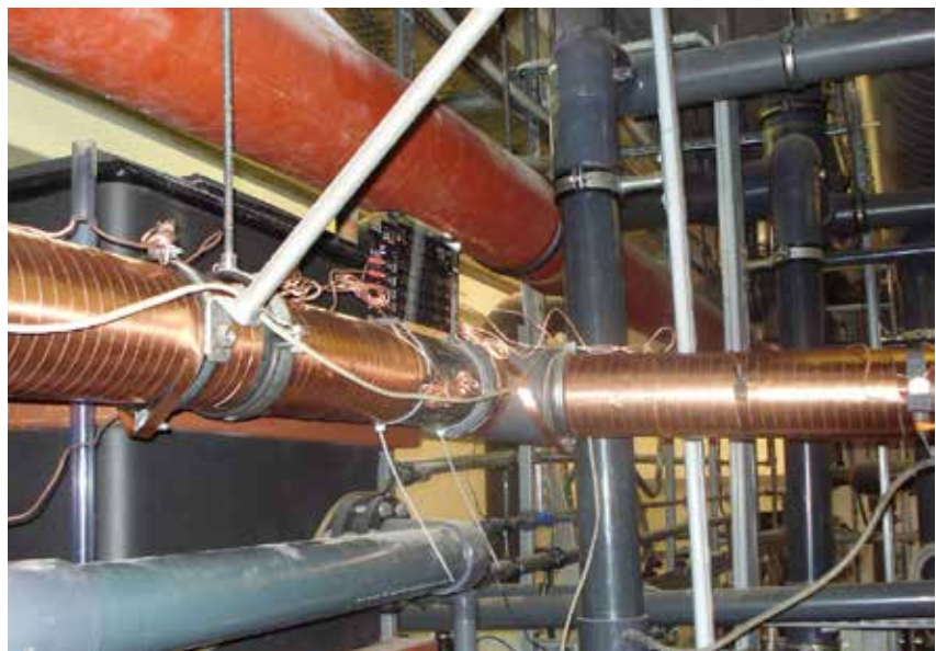
Vulcan S250 treating main water pipes for the Meridan Pool and Spa area
