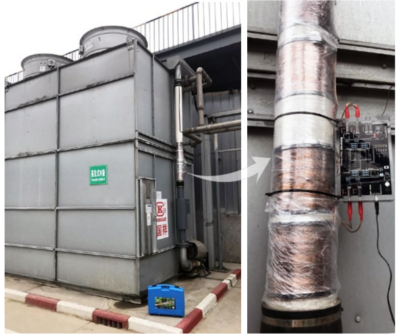
Vulcan S25 was installed at the water inlet of the cooling tower.
