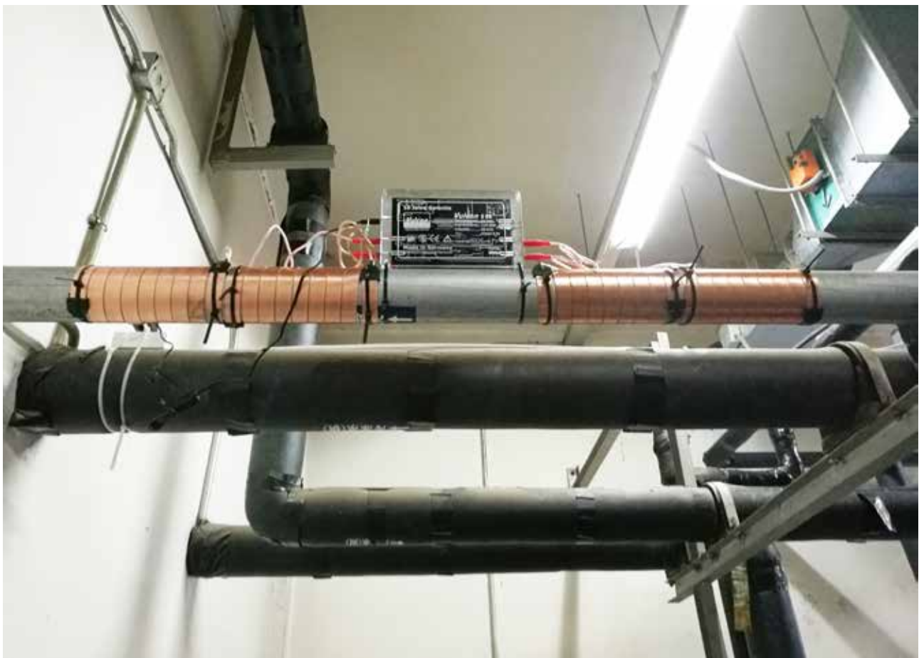
Vulcan S25 installed on the main water pipe of the cooling tower.
